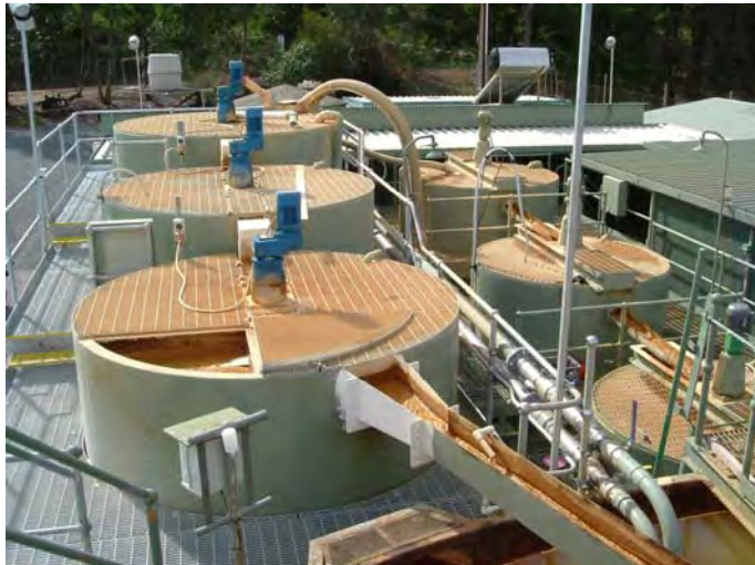
Plate 10. High Density Sludge (HDS) plant used for the continuous treatment of AMD from a decommissioned mine site. Key sources of AMD at the site include pit wall rock and benches, waste rock dumps and a tailings storage facility.
